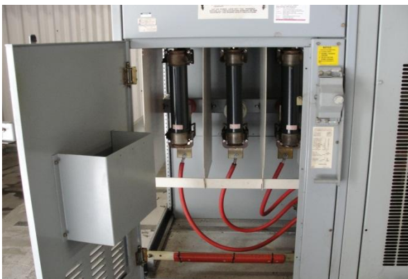
De-energized switch, open front of cabinet for visual inspection
