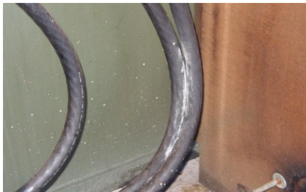
White powder & discoloration on cables
