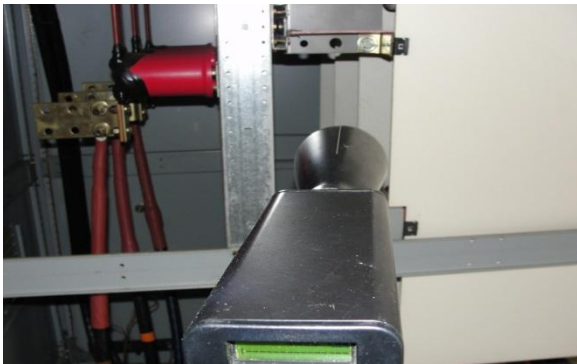
Limited direct line of sight– ultrasound showed noise originating from B-phase fuse stall
