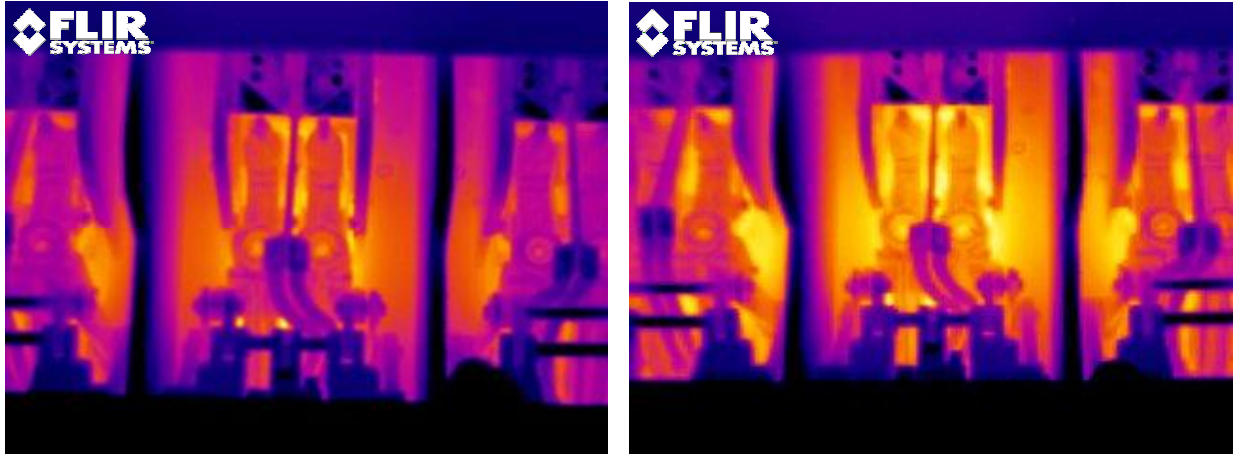
Figure 6. Medium resolution (left) and low resolution IR images of 480 volt generator tie-in breaker.
