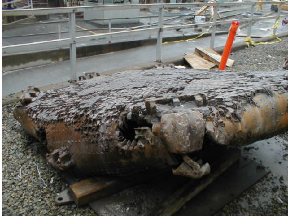
Damaged deflector plate after removal. Note normally straight edges of 4000 lb. steel plate have been rolled over.
