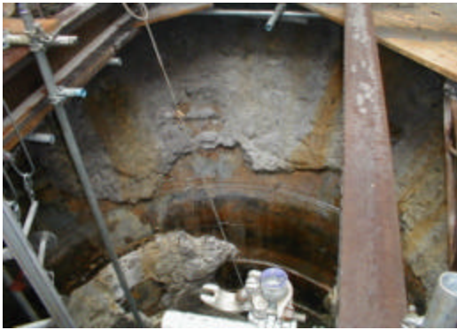
Refractory damage within Regenerator Cone
