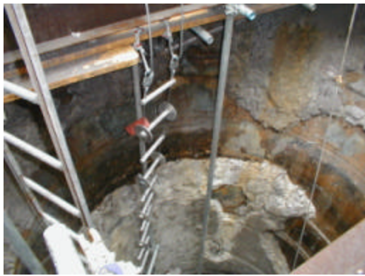
Refractory damage within Regenerator Cone
