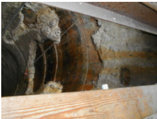
Refractory damage within Regenerator Cone
