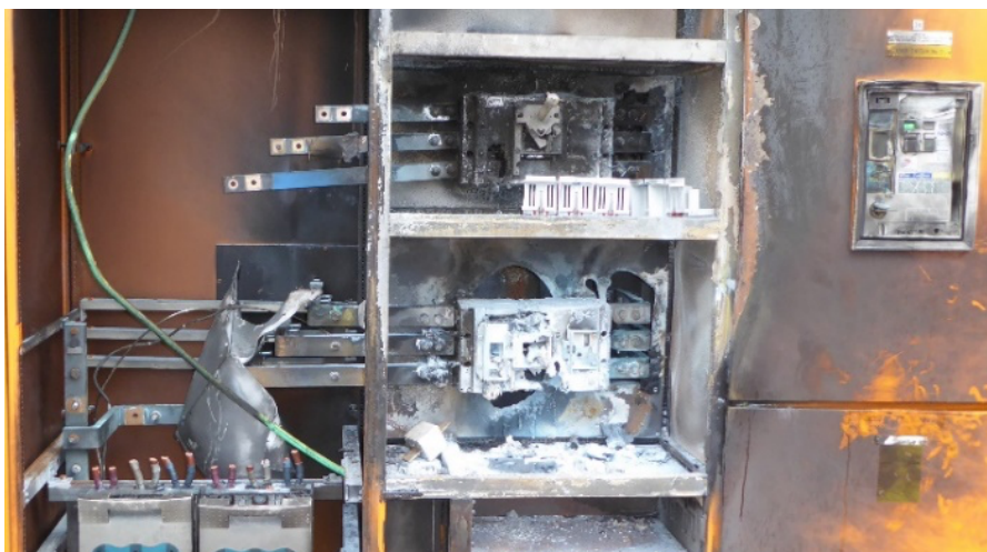
The switchboard was destroyed by the explosion and fire
