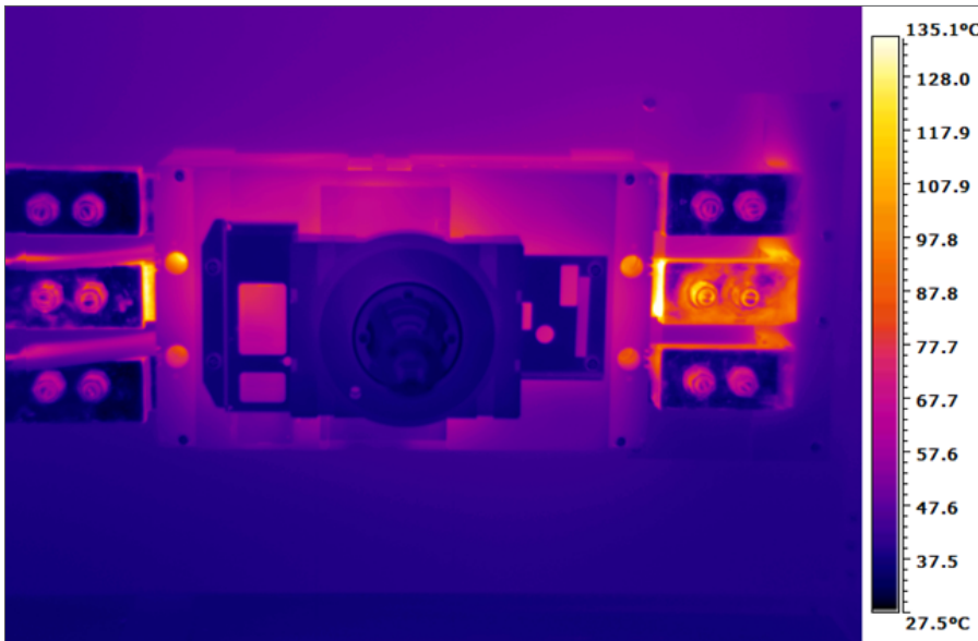
Thermogram of the MCCB before it exploded and caused a fire. Apparent temperature on the RH white phase near the body of the MCCB was 147°C. Apparent temperature on the LH white phase near the MCCB body was 136°C
