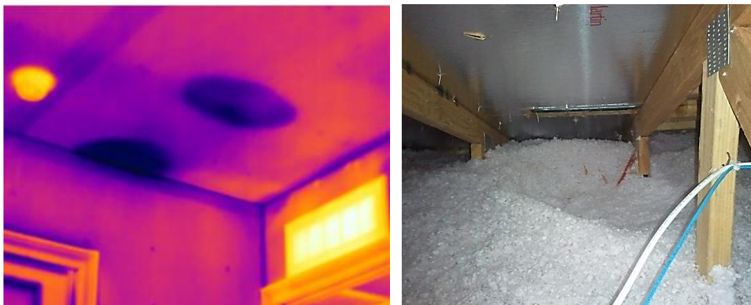
Leak or missing insulation? The image on the left is a leak; however, I have seen similar anomalies with missing loose-fill insulation that occurs in attics when wind is blowing through roof vents which creates a vortex spiral in the insulation.
