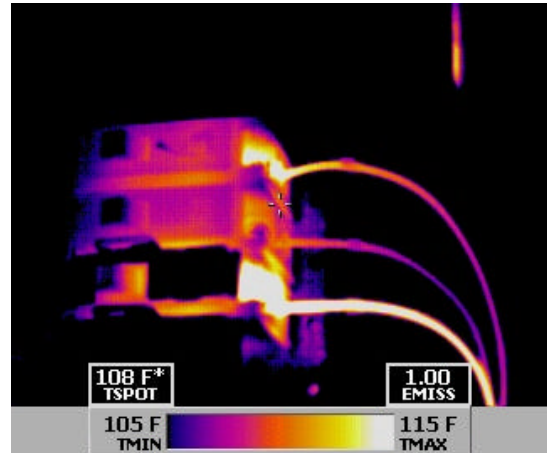
Above thermal image shows overheated conductors on the load side of single-phase, 20 amp breakers.
