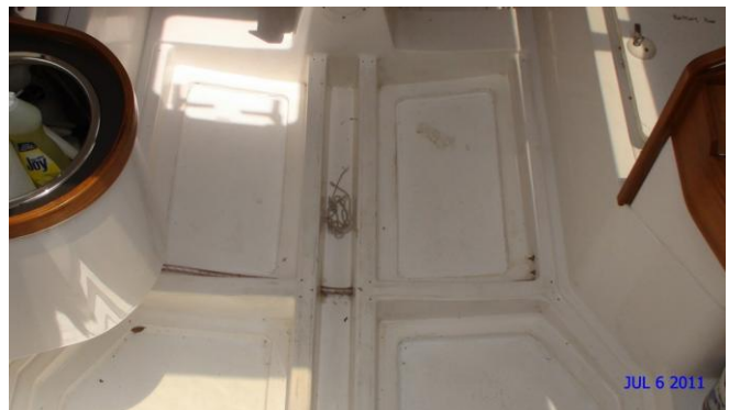
Internals of vessel showed that bilge area above the suspect thermal pattern and elevated moisture meter readings was clean and dry
