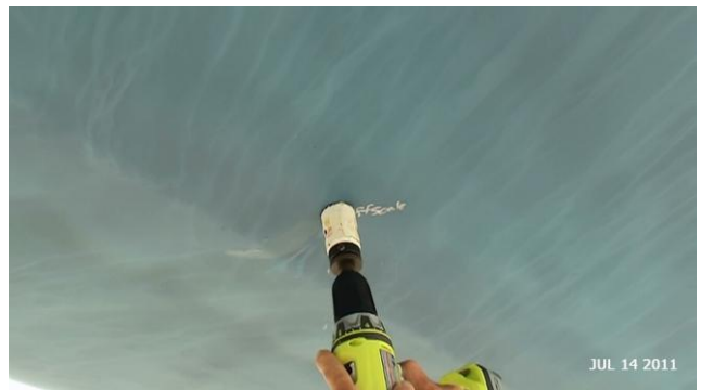
Hole saw attachment on drill used to take core sample for destructive testing
