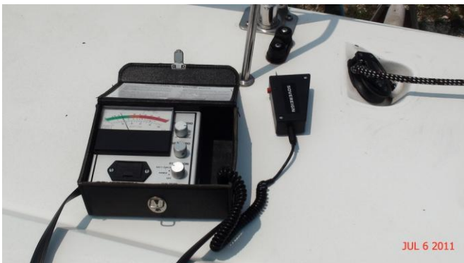
Suspect water intrusion from thermal image detected using capacitance style analog moisture meter
