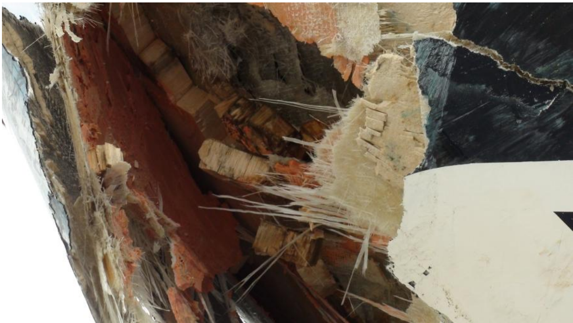
Visual inspection showed topsides were a FRP cored laminate composed of gel coat, layers of fiberglass mat and cloth, bonding paste, balsa core, and layers of fiberglass cloth
