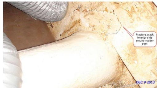
Visual image of interior side of fiberglass laminate surrounding the rudder post shows evidence of fracture cracks, corroborating thermal anomaly
