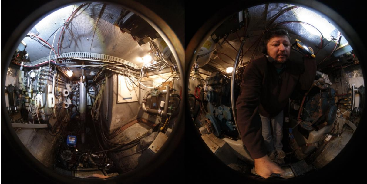
Figure 11. An unstitched view of the confined space for the engine compartment shows two (2) one hundred eighty 180° FOV images before stitching.
