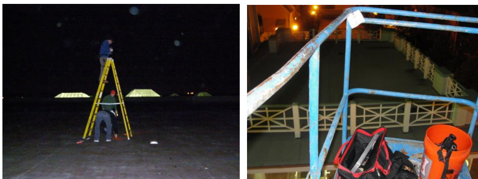
Figures 5: Using ladders and aerial lifts to overcome reflection and hard-to-reach roof areas can be time saving and dictate the success of a job.
