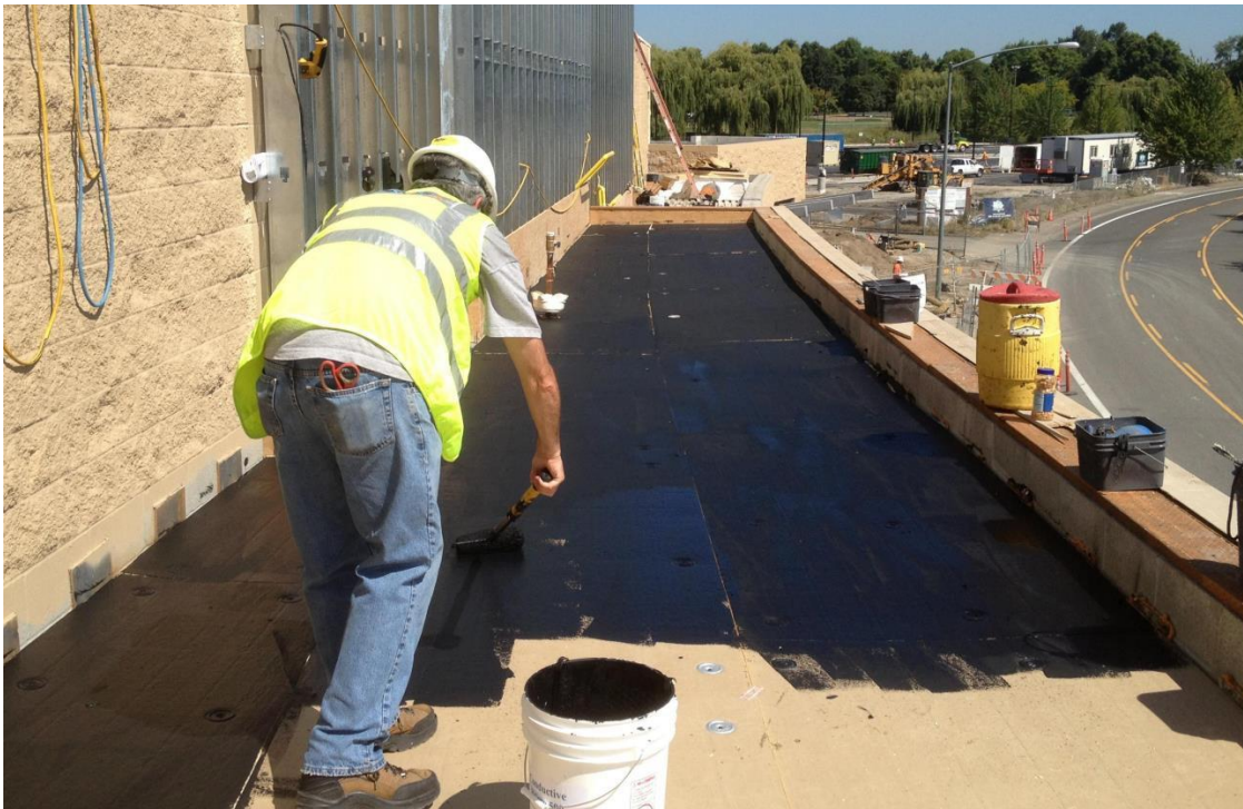
Figure 9 : TruGround conductive primer being applied to a cover board substrate before installation of the membrane.
