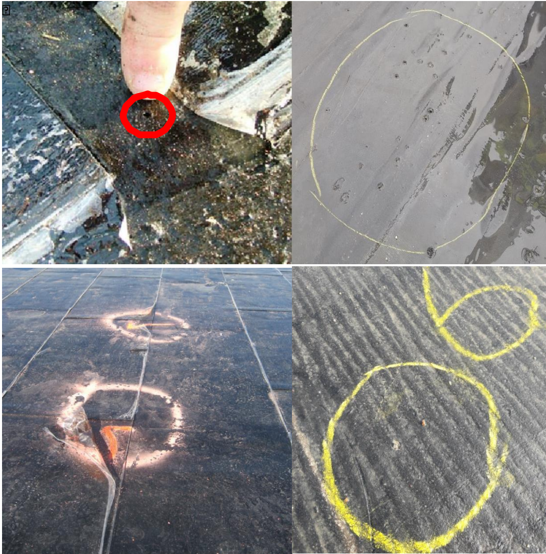
Figure 7: Breaches found in inverted waterproofing/roofing assemblies.
