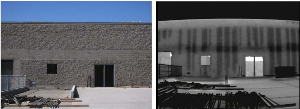
Figure 3. Visual and IR image of CMU building wall. (Grouted areas are lighter.)
