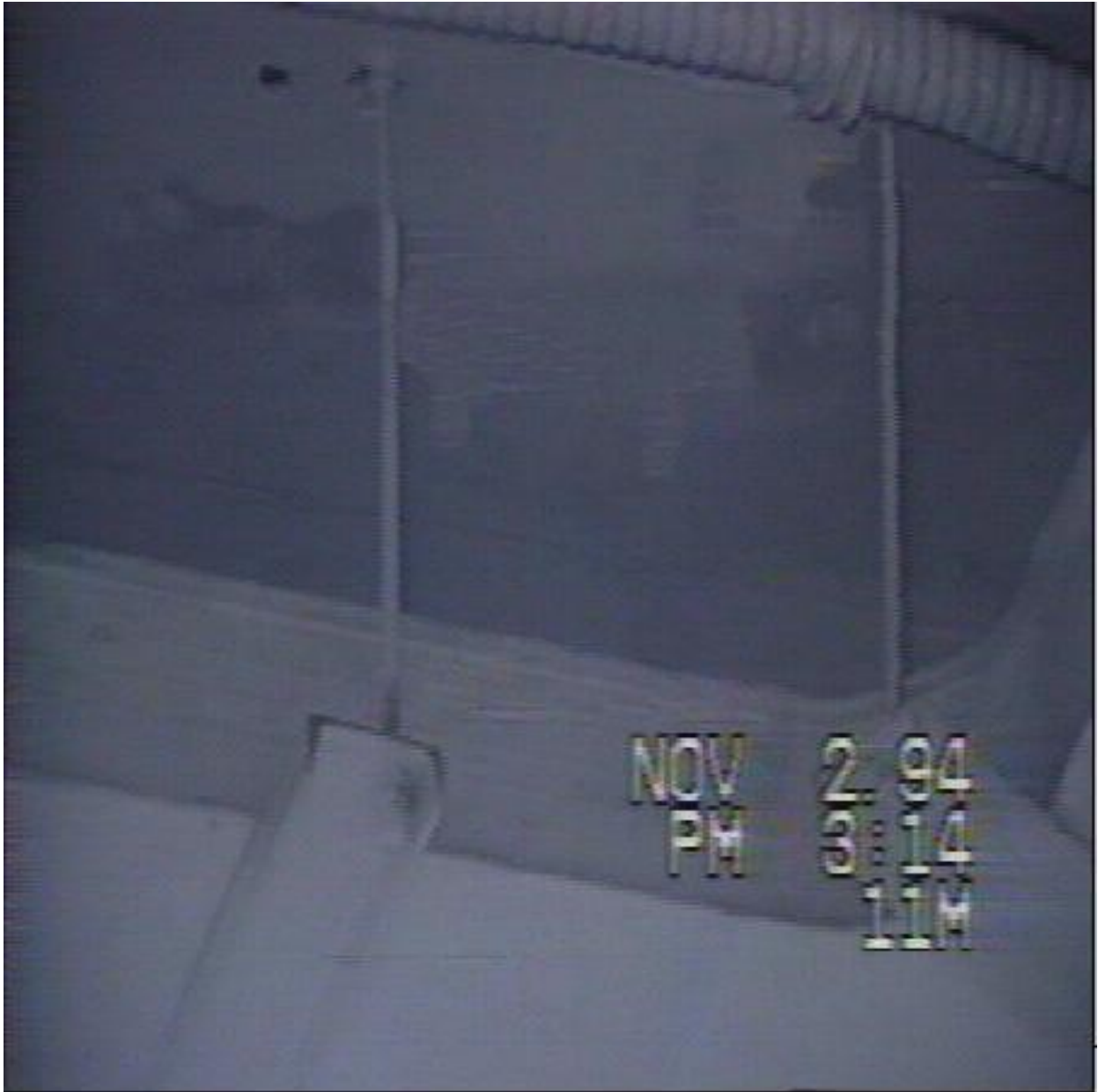
Calvert Bus Duct
