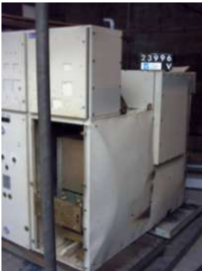
Fig 15. Buckling caused by 20kA arc-flash
