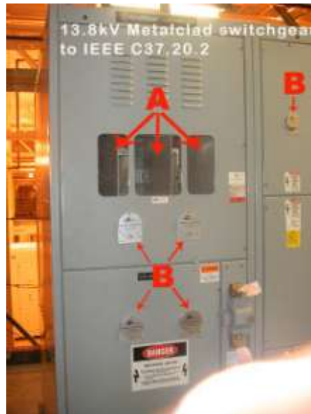
Fig 1. IEEE C37.20.2 compliant cabinet
