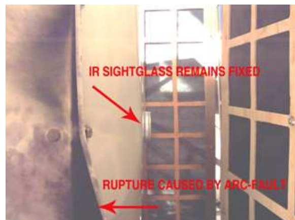
Fig 7. Results of an arc-fault test including IR sightglass installation
