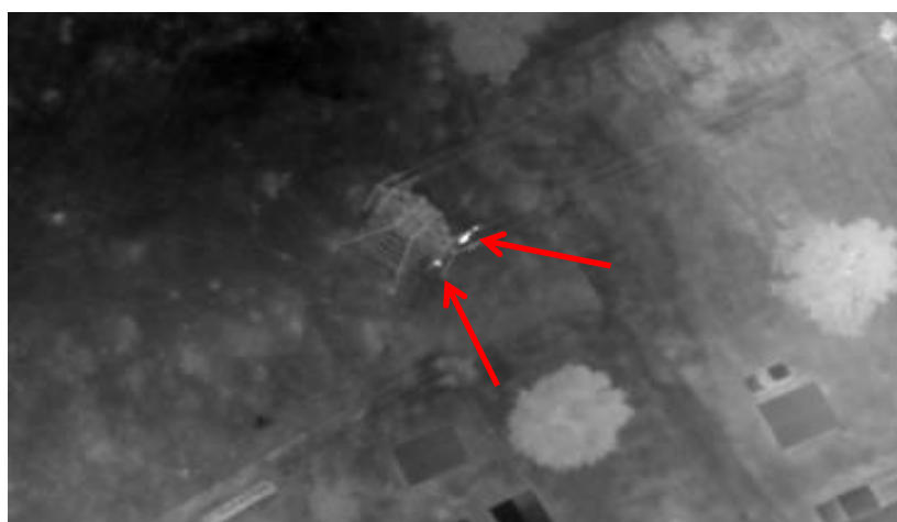
Figure 6. Hot connections on a high voltage transmission line
