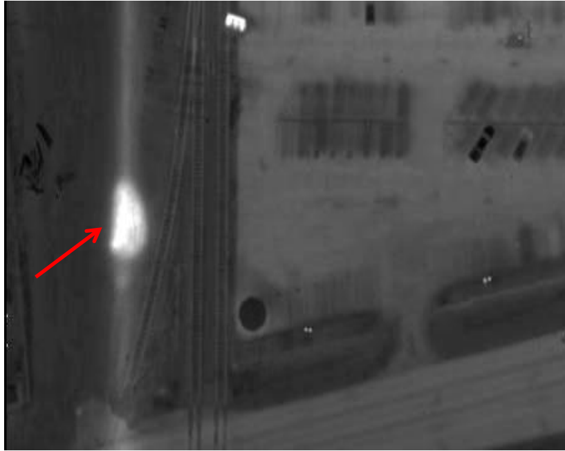
Figure 3. Typical steam leak in a distribution system
