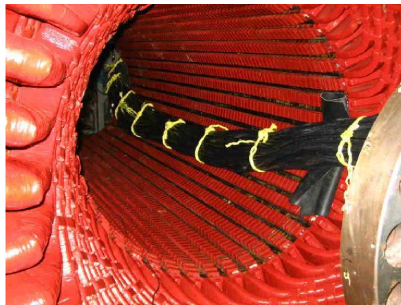
Generator stator core - coils wrapped around and ready for fluxing
