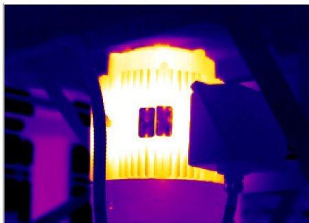
Overheating fan motor due to insufficient cooling air circulation (dirty fan guard)
