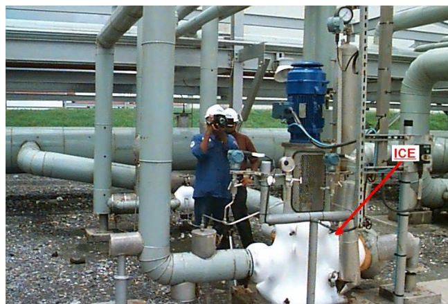
Icing of ammonia line at pump. Ambient air temperature is 35°C (95°F)
