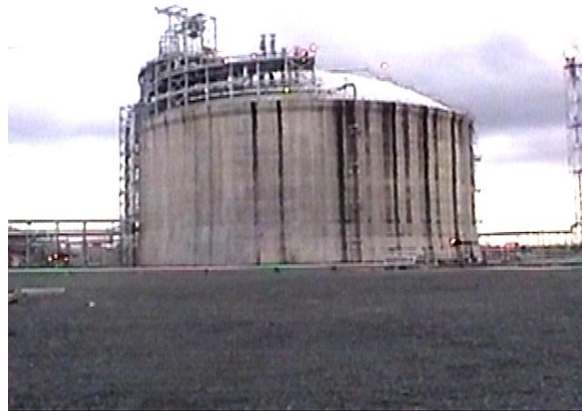
Liquefied Natural Gas (LNG) storage tank with microbial algae and mold growth only on the sea facing side (right side)
