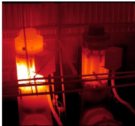
Pump motor on left showing signs of overheating as compared to right pump motor
