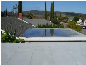
Roof not pitched properly to drain (holding water)
