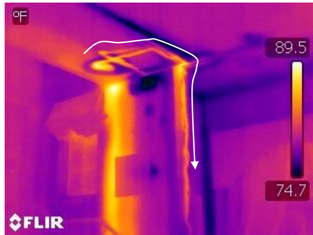
Water testing showing water travel
