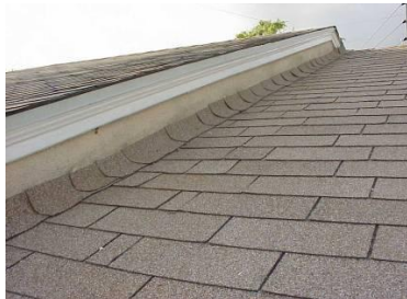
Roof with no proper counterflashing
