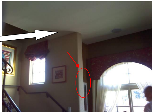
Visual (arrow shows where only visible stain was noted)
