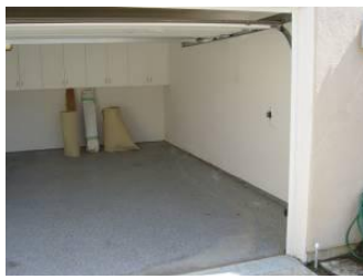
Visual of garage where elevated moisture was noted
