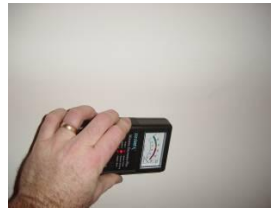
(B) Moisture meter 100% readings
