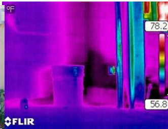
Thermal image showing wet area of wall
