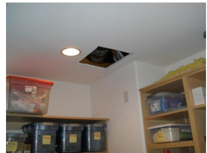
2nd story above bedroom closet suspected and owner cut holes in ceiling looking for source.
