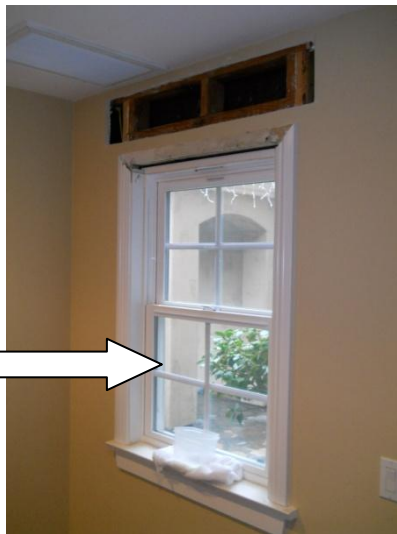
Interior View. Owner opened up portions of wall to find leak.
