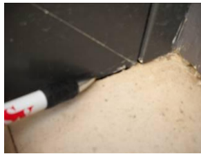
Openings at exterior lacking proper sealant
