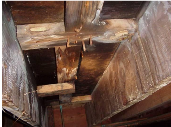
Subfloor damage due to leak
