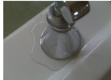
Plumbing fixture leak
