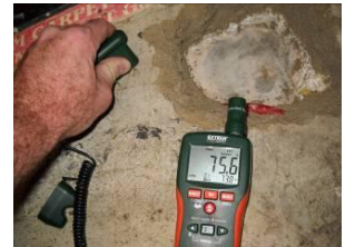
Portions of slab chipped away in areas of high moisture. Notice the red pipe in slab (radiant heating)
