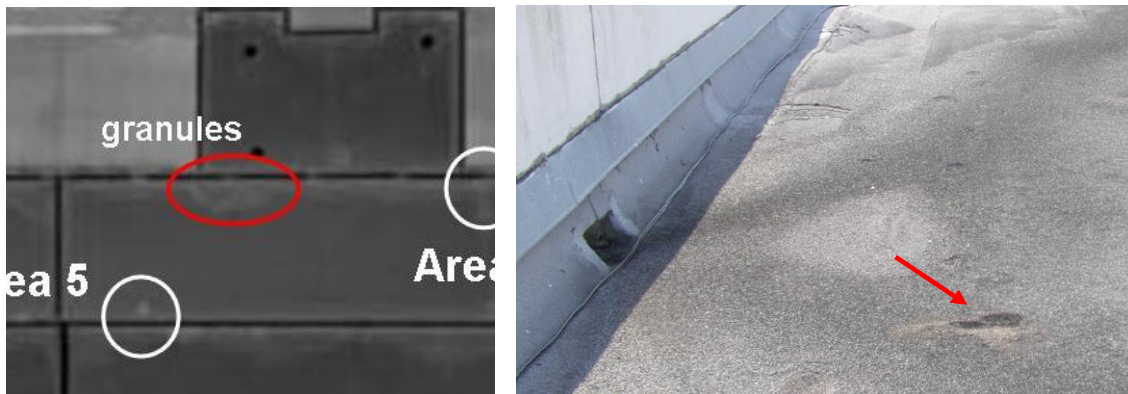
Figure 6: Area of accumulated roof granules (red circle on infrared image) that produced a thermal anomaly observed on the aerial infrared imaging. Arrow in right Figure shows footprint in granule pile
