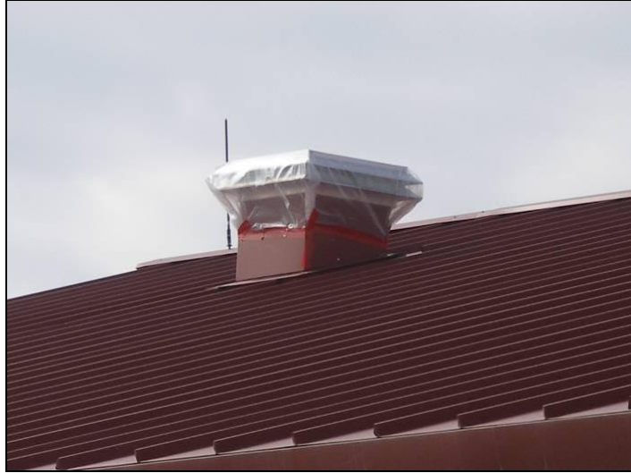
Figure 2. In preparation for an air pressurization test, the exhaust stacks are sealed off as they are understood to be a known or controlled air pathway
