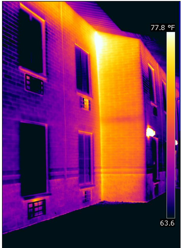
Figure 23. Infrared thermogram showing air leakage at inward corner while enclosure was pressurized
