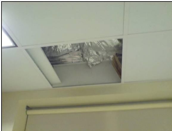
Figure 12. Removed drop-ceiling tile reveals foil faced insulation being used as the formal plane of building enclosure
