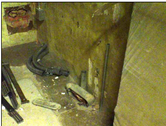
Figure 8. Derelict conduit penetration in concrete slab
