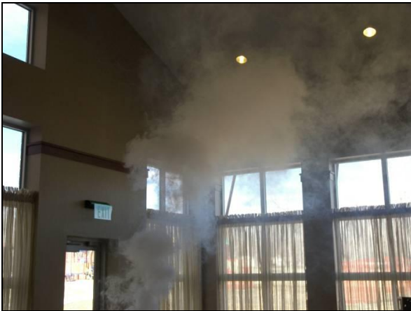
Figure 28. A theatrical smoke machine releases smoke inside the enclosure. When the building was pressurized the smoke could be tracked visually and was found to be exiting through the recessed lighting fixtures
