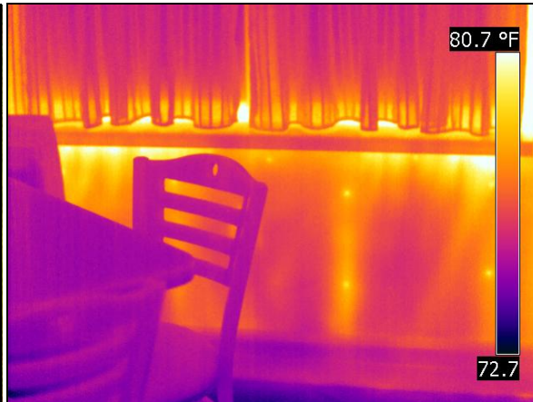
Figure 15. Infrared thermogram reveals air leakage at window sill while enclosure is depressurized
