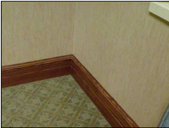
Figure 18. Base trim in a commercial facility with exterior wall on the right and interior wall across the top/left
