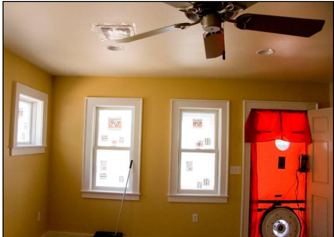
Figure 5. Single fan units can be used to pressure test residential properties
