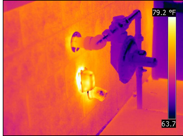
Figure 27. Infrared thermogram reveals air leakage at the electrical penetration while building was under pressurization
