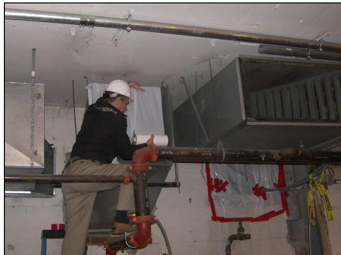
Figure 3. In renovation work, the sealing of existing ducting pathways needs to occur
