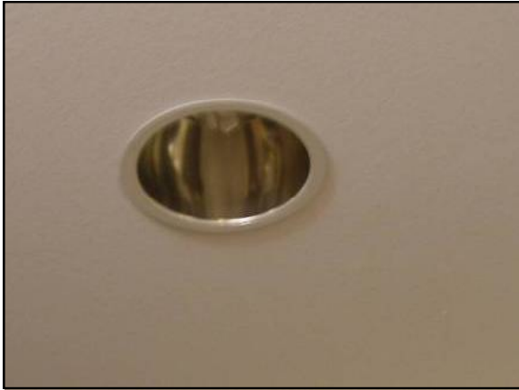
Figure 16. Recessed light penetrating the ceiling GTB that was intended to be the air barrier
