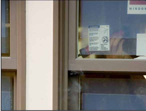
Figure 30. A smoke puffer is used to verify air leakage at a window assembly
