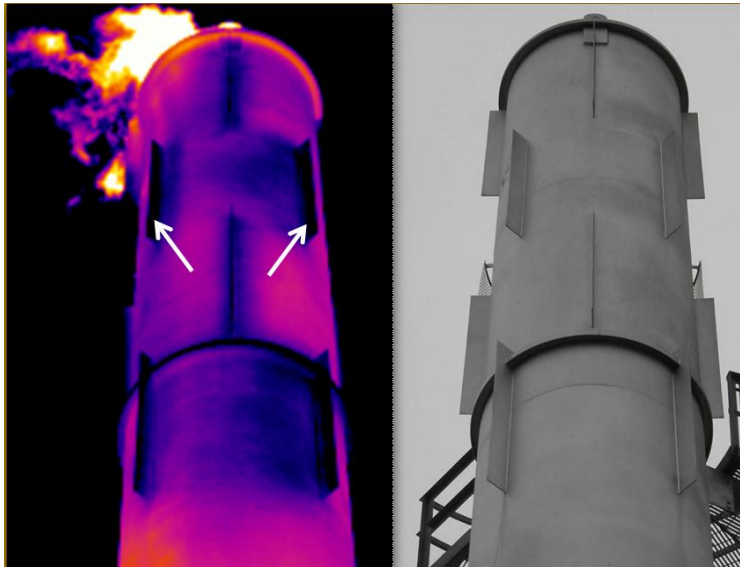
Scrubber Stacks – Factories
