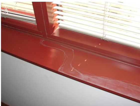
Figure 7 (left): Water stains on window sill.
