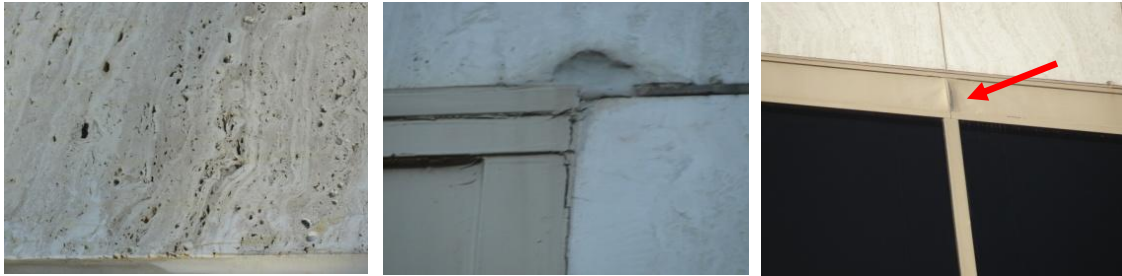
Figure 4 (left): Close-up view of an exterior building tile showing alternating layers of smooth and rough limestone. Some of the dark cavities are deep and may penetrate the entire thickness of the tile.
