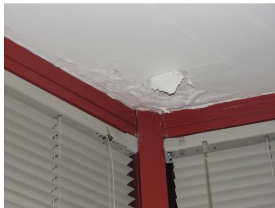
Figure 8 (right): Damaged ceiling on a mid-level floor of the building.
