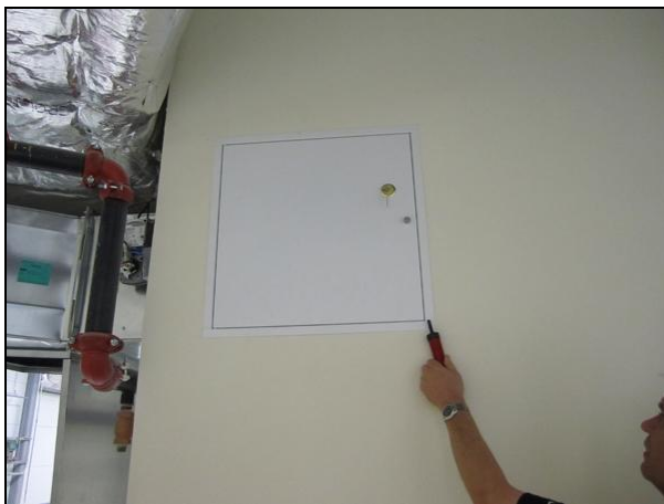
Figure 64. Air leakage was observed through the access door in the mechanical penthouse wall
