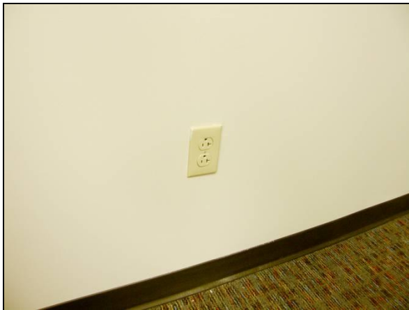
Figure 10. Interior wall outlet
