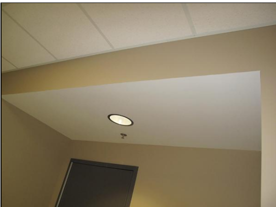
Figure 16. Recessed light penetrating the ceiling GWB that was intended to be the air barrier
