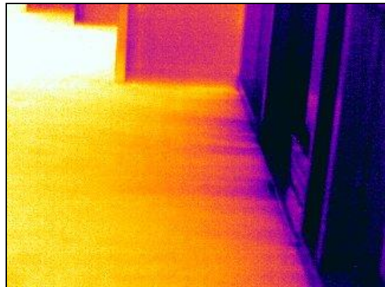
Figure 21. Infrared image showing air infiltration under the exterior storefront doors during depressurization
