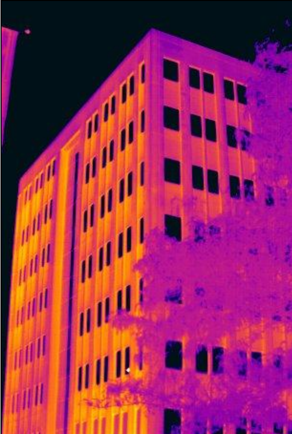
Figure 50. Infrared image of the Southeast corner of the building showing no thermal
