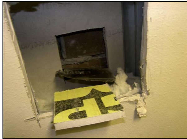
Figure 31. Invasive investigation reveals actual as-built conditions. Additionally, as each material is carefully excavated a pressure differential can be measured between material planes which helps to understand the root cause of failure in a forensic investigation of an air barrier system
