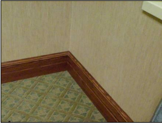
Figure 18. Base trim in a commercial facility with exterior wall on the right and interior wall across the top/left
