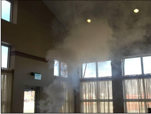
Figure 28. Theatrical smoke machine releases smoke inside of the enclosure. When building was pressurized the smoke could be tracked visually and was found to be exiting through the recessed lighting fixtures
