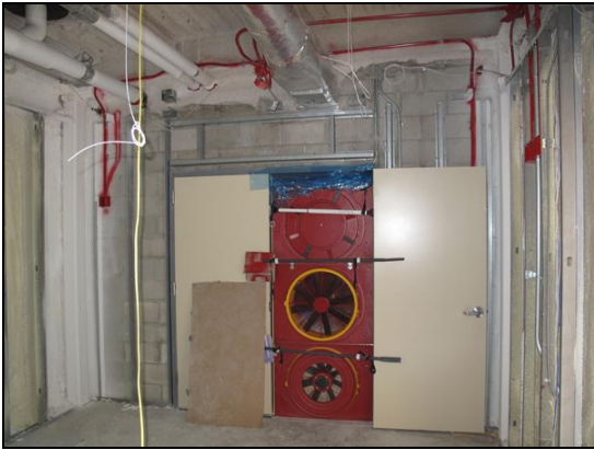
Figure 32. Door fans set up in the South connection to the adjacent building
