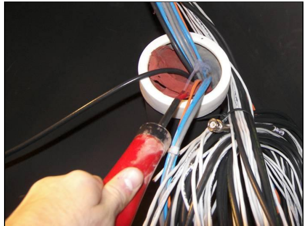
Figure 29. A smoke puffer is used to track air leakage through an audio/visual cable conduit revealing a not so obvious short circuit for air leakage
