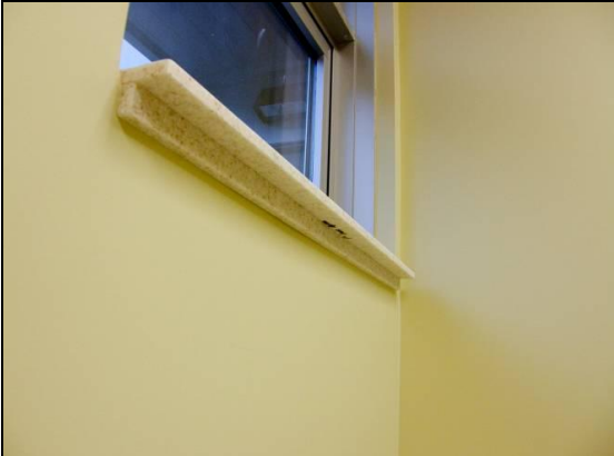
Figure 14. Window sill in a commercial facility
