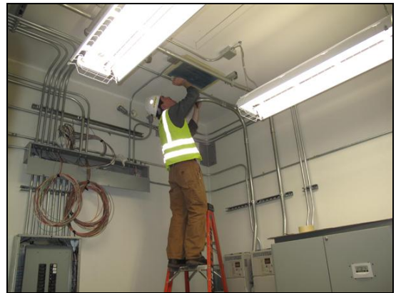
Figure 3. Some vents are more easily sealed from the interior
