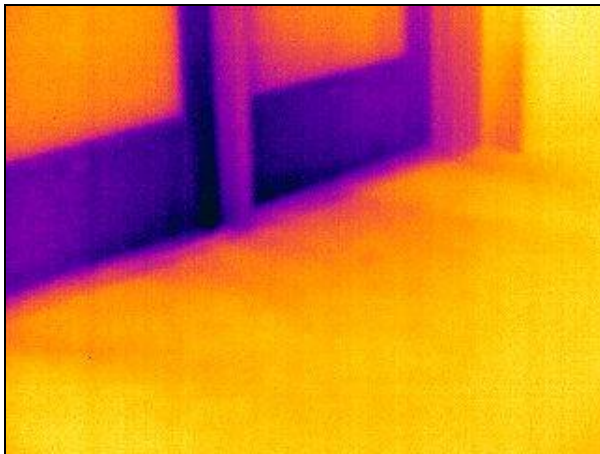
Figure 62. Infrared image showing air leakage around an exterior door in the South building connection
