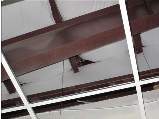
Figure 12. Underside of the super saver insulation scrim in a pre-engineered metal building
