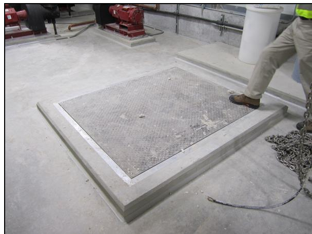
Figure 65. Air leakage was observed through the equipment hoist hatch in the mechanical penthouse slab
