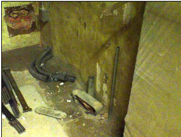
Figure 8. Derelict conduit penetration in concrete slab
