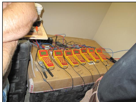
Figure 37. Data acquisition units that relay to the computer station
