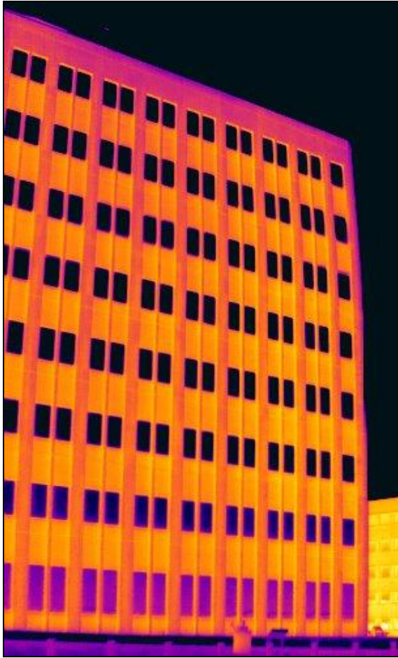
Figure 48. Infrared image of the Southwest face of the building showing no thermal anomalies
