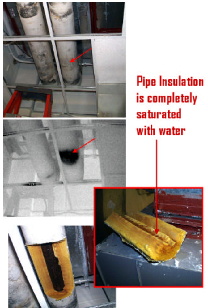
Fig. 5-Wet insulation on cooling pipe system in building
