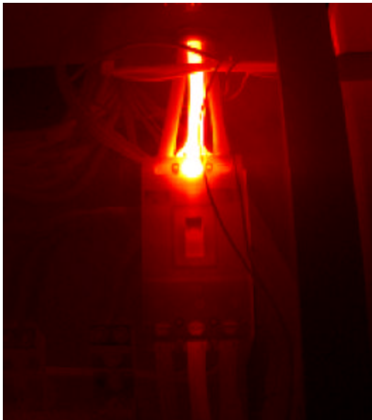
Fig. 1-Loose lug connection on electrical circuit breaker
