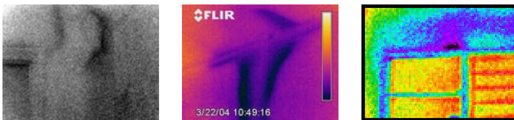
Formosan subterranean termite shelter tubes seen in IR
