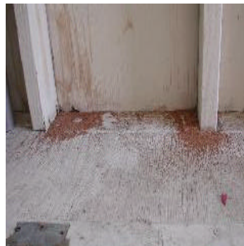
Drywood termite droppings
