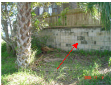
Retaining wall cracked
