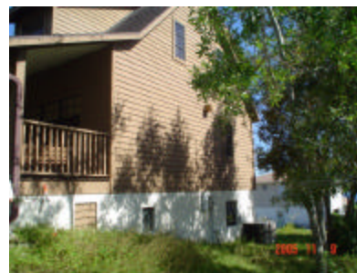
No access to entry of crawlspace
