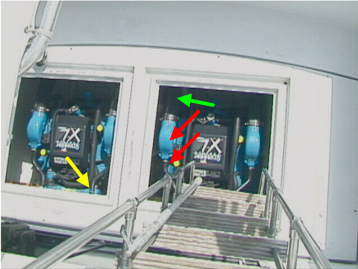
Figure 1. Looking down from above into the engine compartment. Here are two gasoline powered engines. Each engine has an open (raw water) and closed water cooling system. The raw water system takes the water that the boat is floating in, passes it through a heat exchanger (yellow arrow) for the closed water cooling system. Then, raw water mixes with combustion exhaust gases at the exhaust manifold (red arrows) and routes the cooled exhaust gases and raw water mixture overboard (green arrow) through an exhaust hose.
