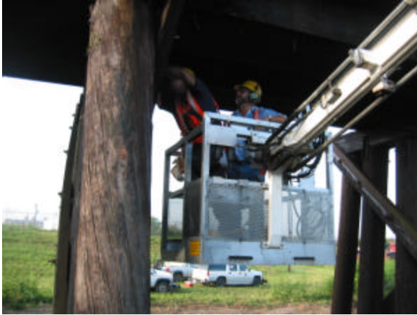
Digital image at left shows the piling and caps structure being inspected in Section C.
