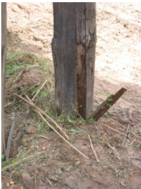
Manual and visual inspection of the piling revealed evidence of mud tubes and physical damage.
