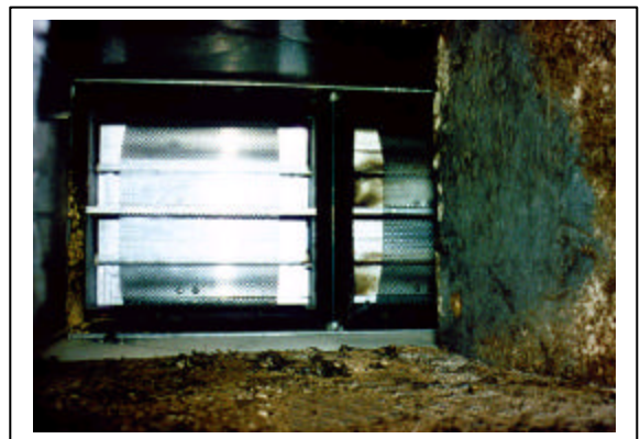
Mold in HVAC ductwork.
