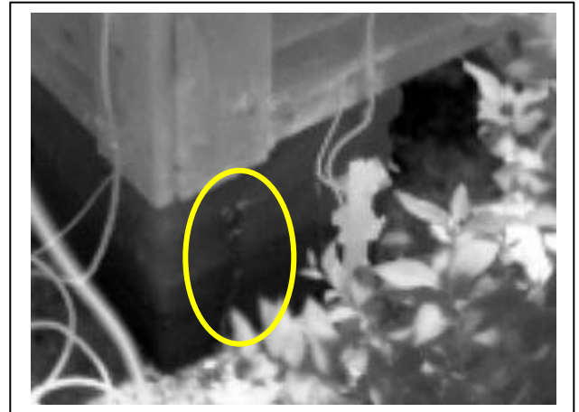
Termite mud tube on pier blocks – Orlando, FL
