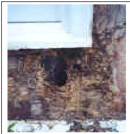
Water and termite damage at windowsill with EIFS insulation (EIFS removed)
