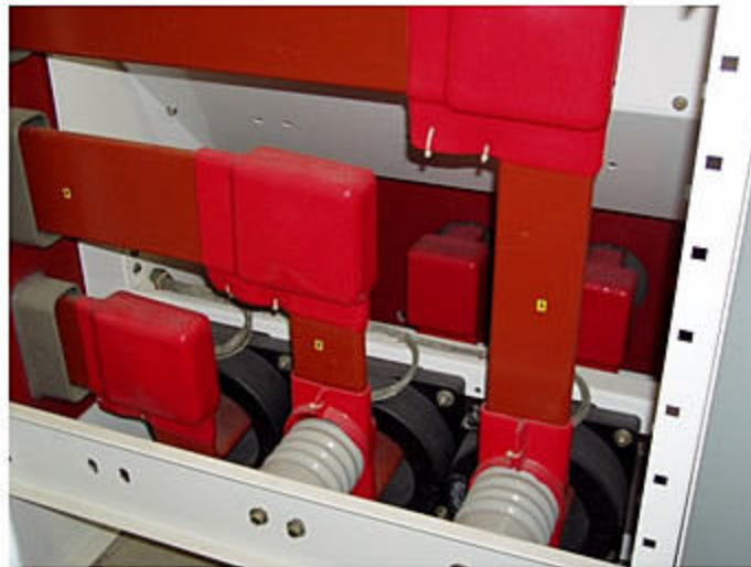
Back side of cabinet showing stationary contacts
