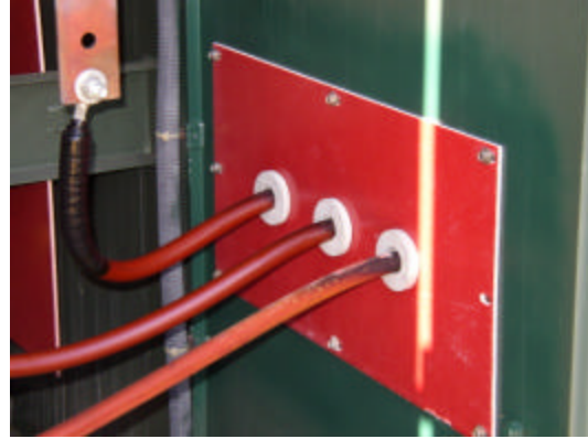
Figure 5: Non-shielded 23kV cables in contact with grounded porcelain collars produce corona conditions. Note discoloration of cable in foreground.
