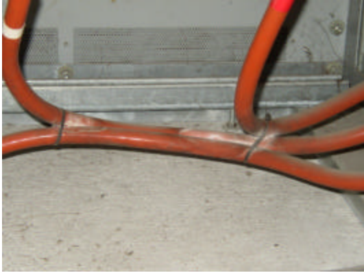
Figure 4: White powder/dust residue formed on 13kV power cables that are tie-wrapped together, forming tight air spaces between each other; ideal locations for corona to form.
