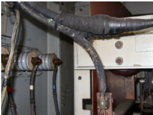
Figure 6: Severely deteriorated power feed cable in 4160V switchgear cabinet displaying white power and carbon tracks
