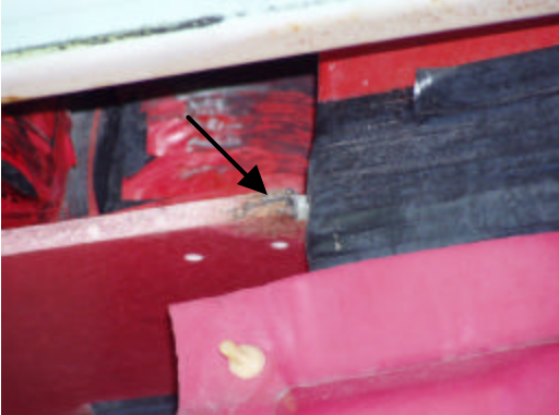
Figure 2: Corona tracks on insulation board close to 13kV bus bars
