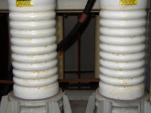
Figure 3: Contamination on ceramic bushing caused corona discharge to form
