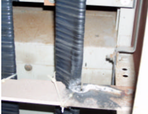
Figure 1: Advanced stage of carbon tracks on insulation board and insulated tape wrap on 4160V bus
